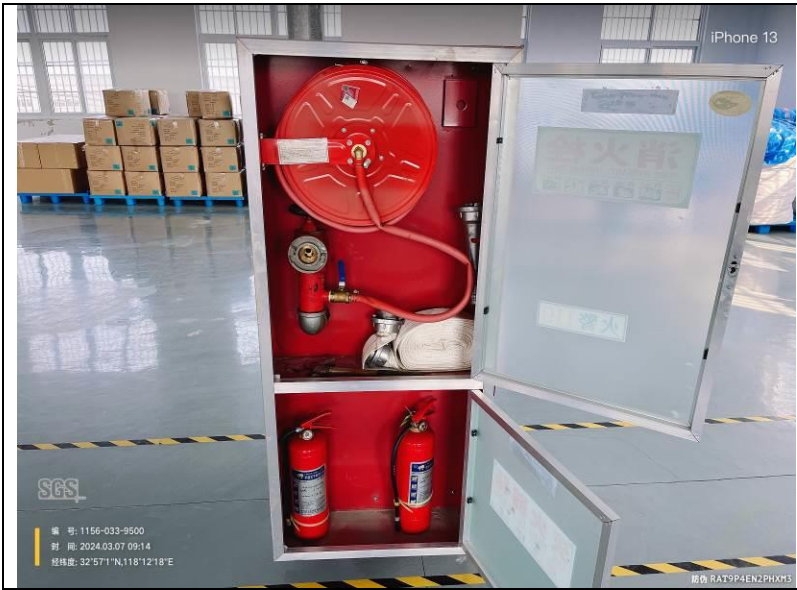
Fire hydrants and fire extinguishers
